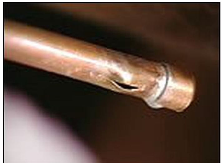
Frozen Copper Pipes will bulge and split
